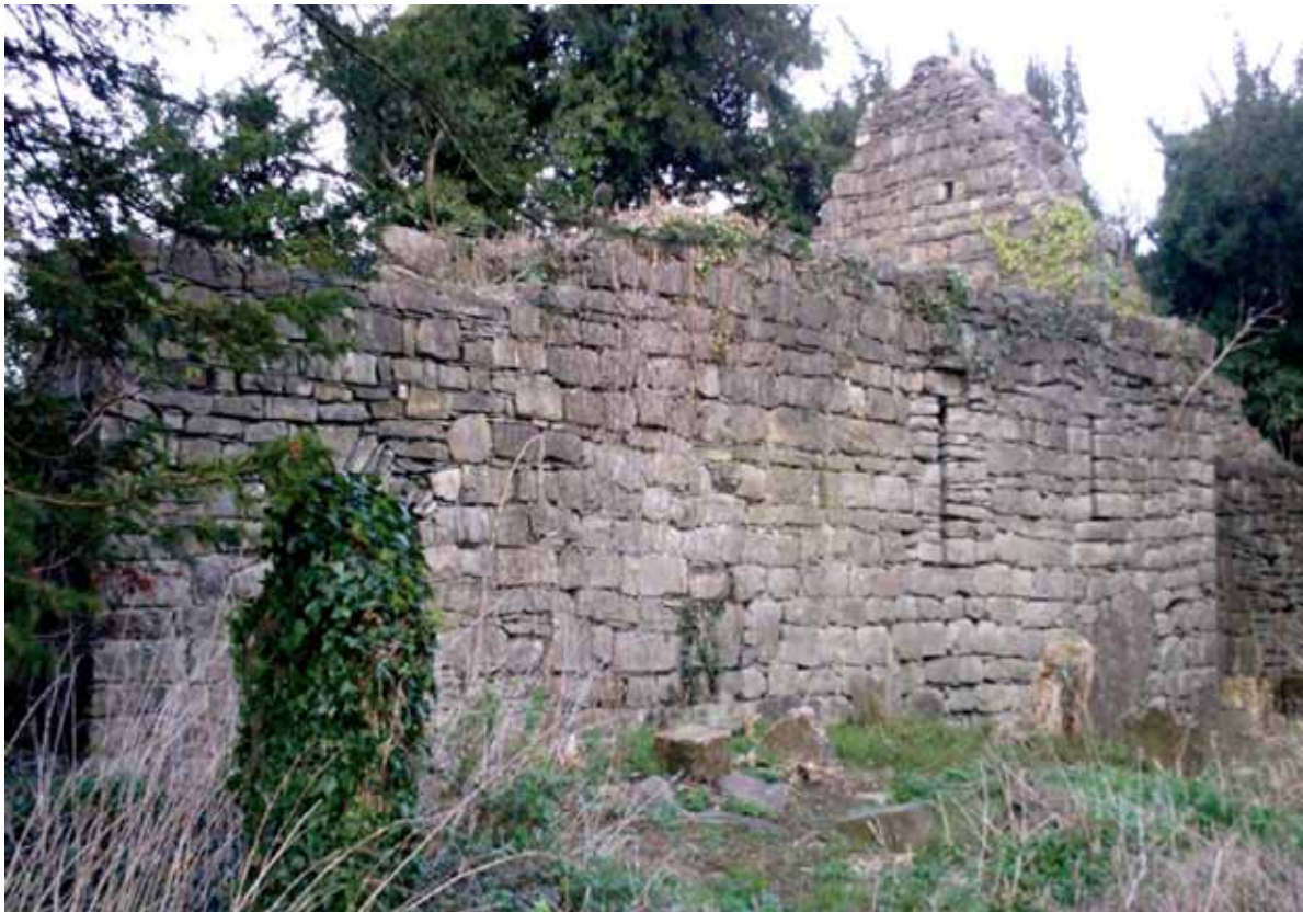
The Confey church was built as a single-celled structure but the chancel was added about a hundred years later.
